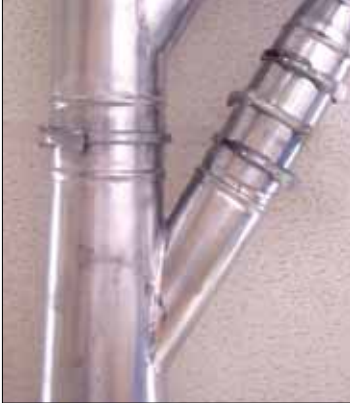
Example of metal ducting specifically designed for dust collection.
